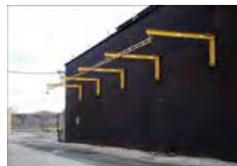
SPANCO Rigid Lifelines Fold-Away Fall Protection system that was mounted to the outside of an existing building structure.
