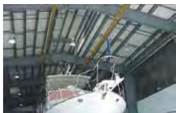
Two SPANCO Ceiling Mounted Fall Protection systems are used to protect workers as they climb on top of large yachts.
