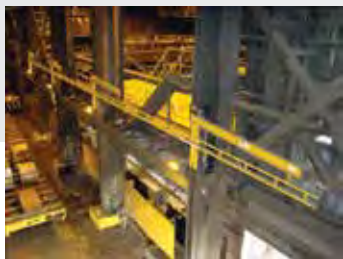
SPANCO Rigid Lifelines Fold-Away Fall Protection System with optional motorization inside of a steel furnace bay. System shown in closed position. System utilizes dual track design, allowing two employees to pass each other without detaching from the system.
