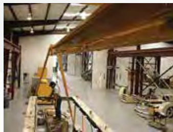
SPANCO Portable Gantry Fall Protection system used inside a large generator fabrication plant. Rolling portable gantry's gives the ability to use as needed.
